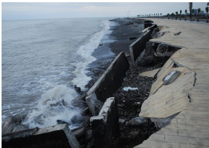
Figure 3. Eroded Boulevard of Batumi
